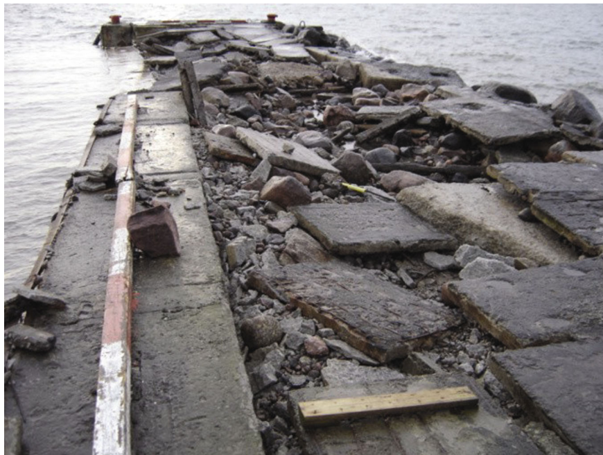
Fig. 3. The damage caused to Aegna Harbour by the storm in January 2005 (Photo by H. Udusaar).
