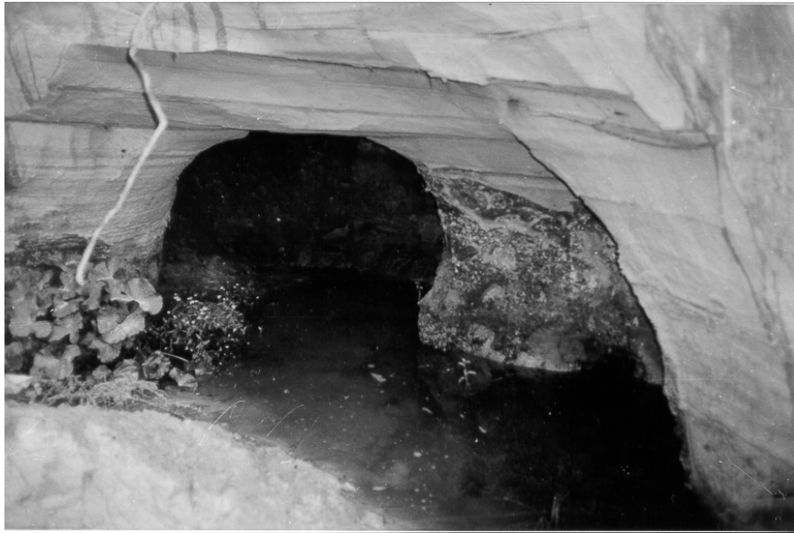
Fig. 5. Visible connection with fractures disappears as the cave widens and a round arch-like bearing is formed.
