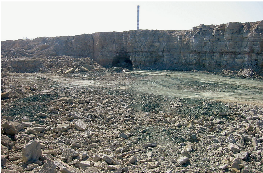
Fig. 9. Consolidation of the Sillamäe uranium mine using the earthworks method. The whole mine area in the foreground is excavated down to the mine floor, and coarse material is placed back to fill the area on the far left. Photo: Kalmer Sokman.
