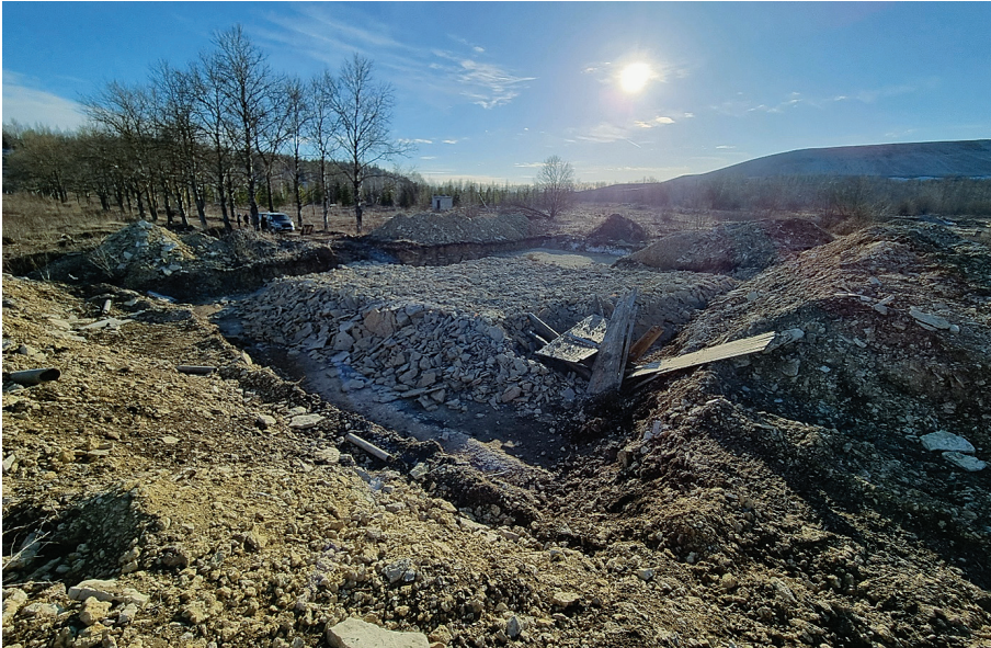
Fig. 10. Stabilization of land above a shallow mine using the blasting method. Test site after blasting pillars at the mine level and strata above the mine roof. Photo: Hendrik Klaas.
