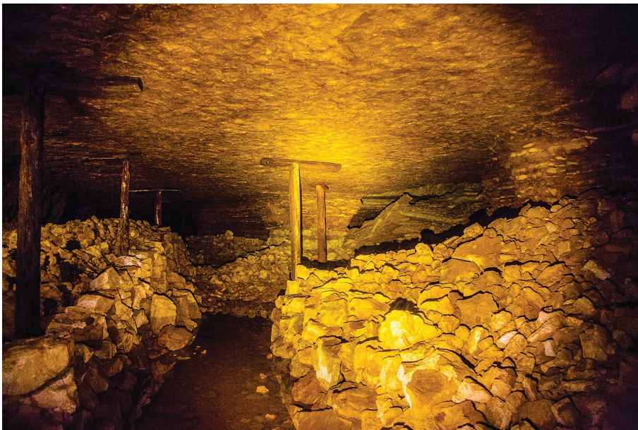
Fig. 8. Partial backfilling with manually laid limestone supports in an Estonian longwall mine, a common practise at the beginning of industrial mining. Note that the supporting rock piles do not reach the mine roof. Photo: Urbex Estonia.
