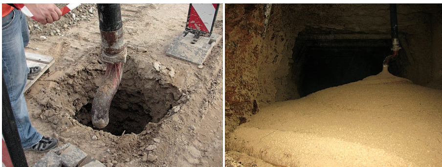
Fig. 11. Stabilization of the addit in the Kukruse mine using the backfill injection method during road construction. Photo taken both from the ground level and from inside the addit during ongoing backfill injection [13].
