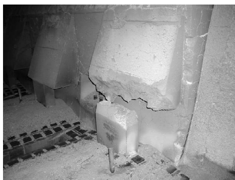
Fig. 4. Disintegrated refractory of canopy (position 1, Fig. 2).
