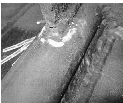
Fig. 3. Penetrating crack on tube walls (position 2, Fig. 2).
