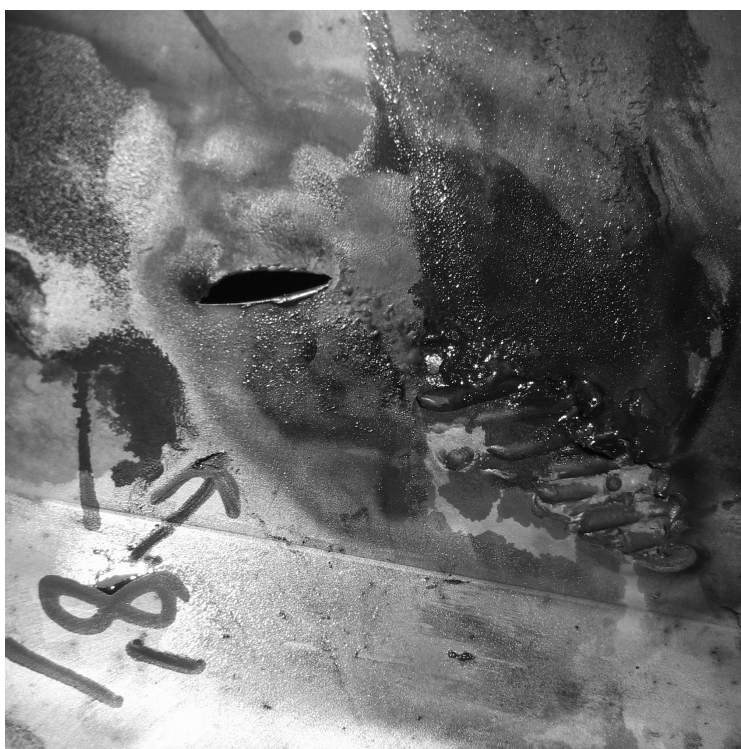
Fig. 2. The penetrating hole in the chute of the fuel supply canal.
